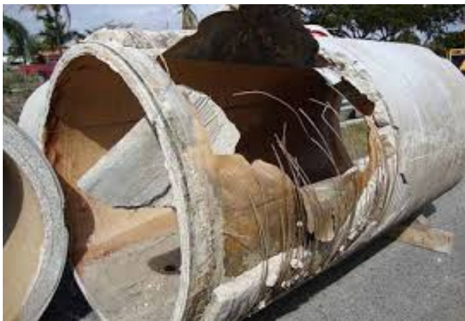
Photo 3: This is another PCCP pipe failure caused by either defective installation or defective manufacturing. Either way, it was defective from day-one.
