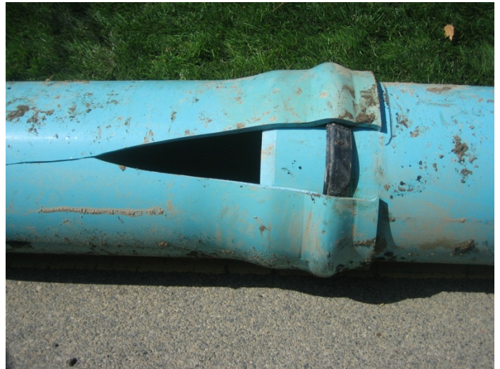
Photo 2: Split PVC C900 pipe caused by either defective pipe material or poor installation. Either one is a day-one defect.
